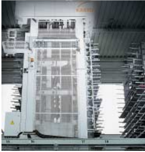
Operating crane in gantry design with maintenance catwalk.
